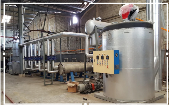
Oil/Gas Fuel Thermal Oil Heater
